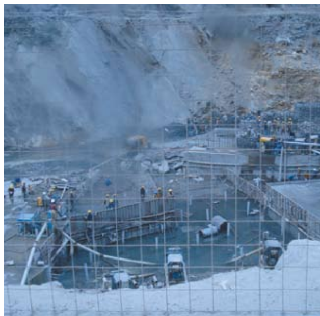
Construction of the 600 MW Loharinag-Pala Hydropower Project on the Bhagirathi River in Uttarakhand, India, 2008. Photo: Matu People's Organization
